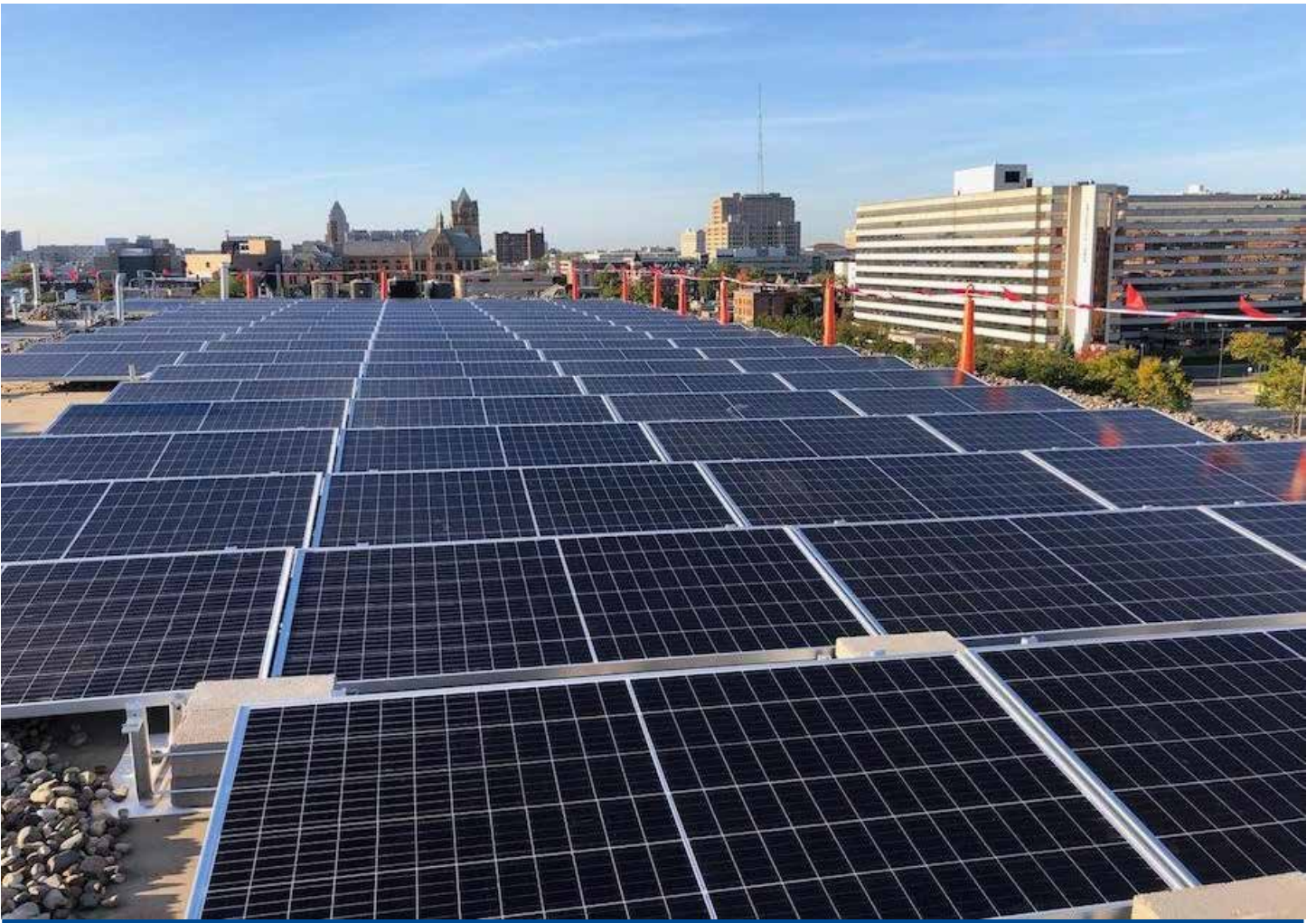
Solar on a former Jeep factory in Detroit.
